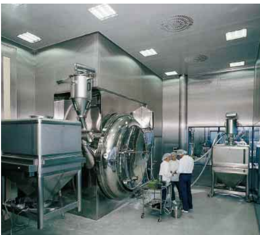
Pharmaceutical cleanroom with Viledon HEPA filters
